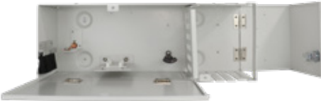
Indoor Fiber Distribution Hub (Open)
